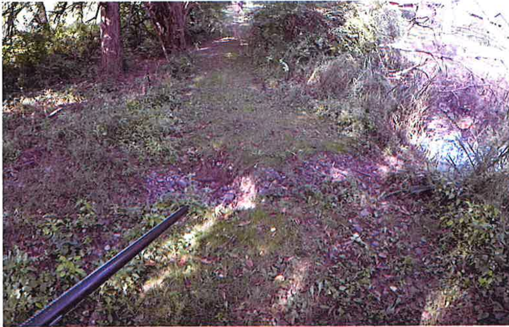
Photograph 3: Beginning of Rip Rap Overflow from Retention Pond #1 to Gumwood Road Retention Pond
