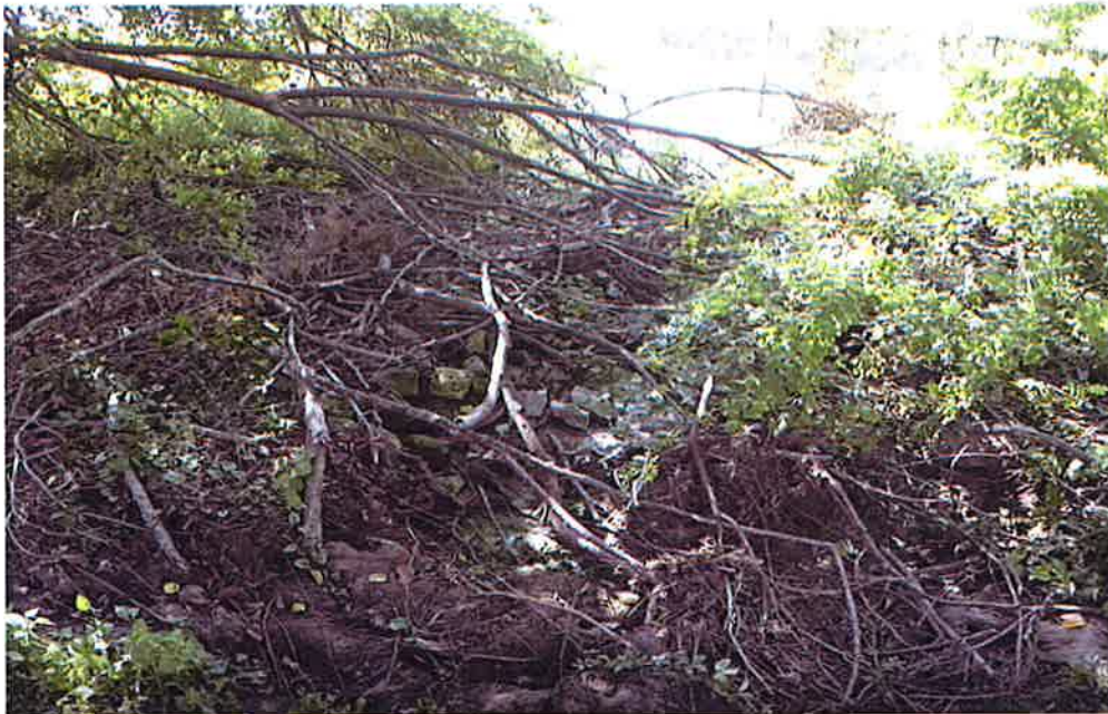
Photograph 4: Rip Rap Lined Overflow from Retention Pond #1 to Gumwood Road Retention Pond
